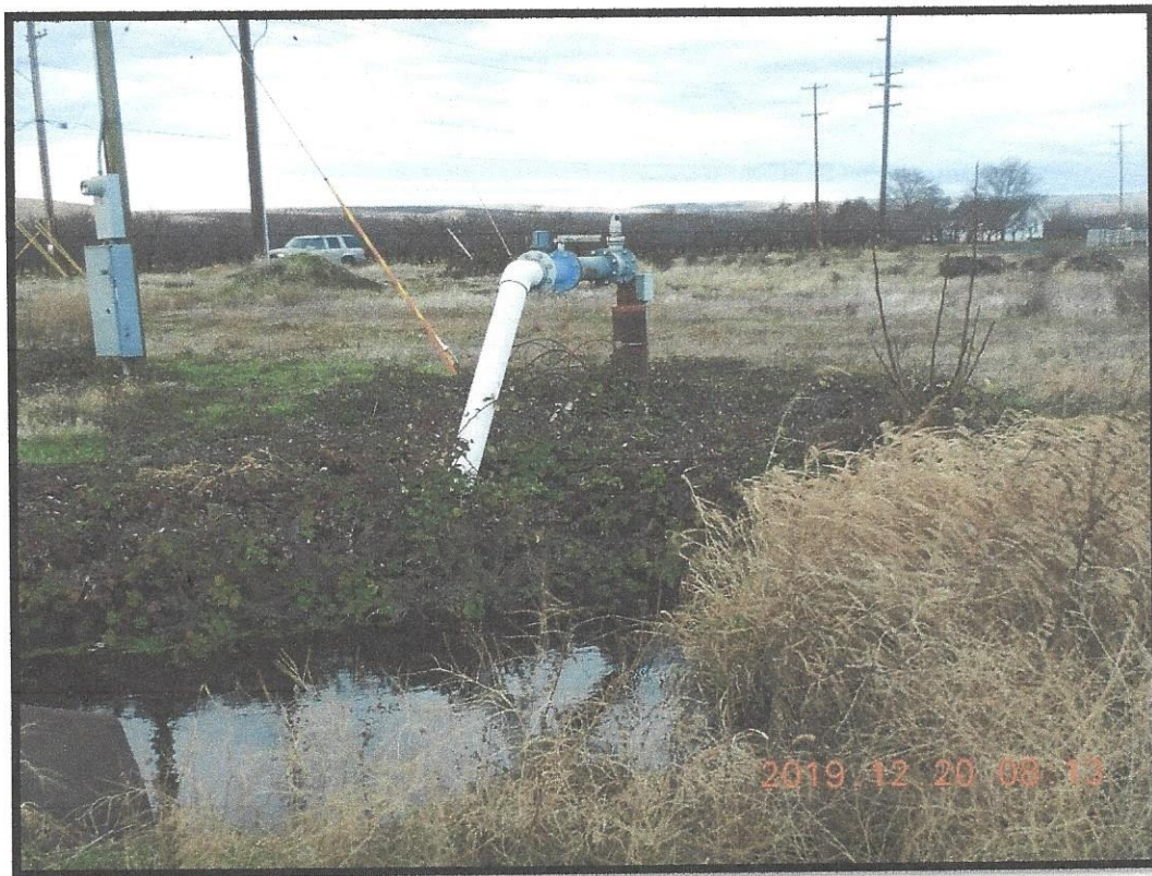
Figure 4 – Looking southwest at the well that will be tied into for the sprinkler system’s water supply. The irrigation system will be connected to the well on the northeast side of the ditch, away from the well.
