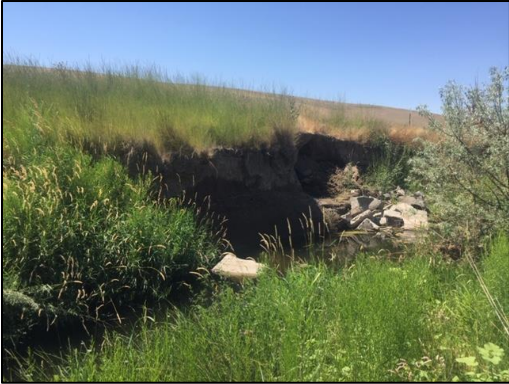
One area of the reach where there is heavy degradation and incision of the channel. There are a few other spots that have similar size incisions.
