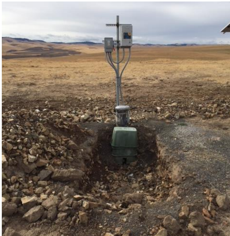
Closer view of well pump
