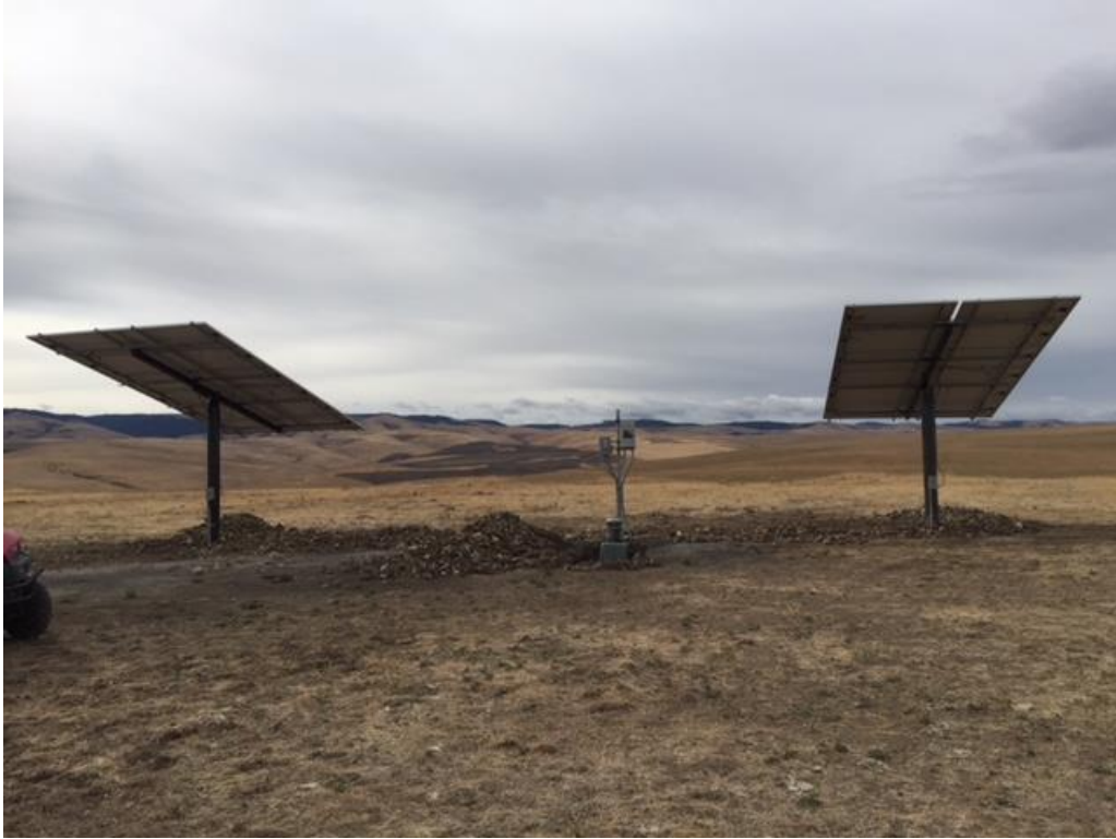
Well pump and solar panels around which a fence will be installed
