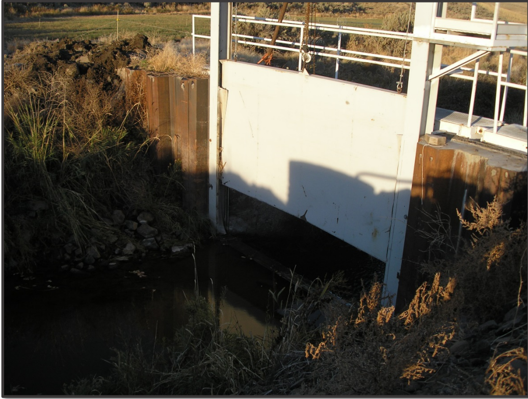
Existing POD where sump is installed.
