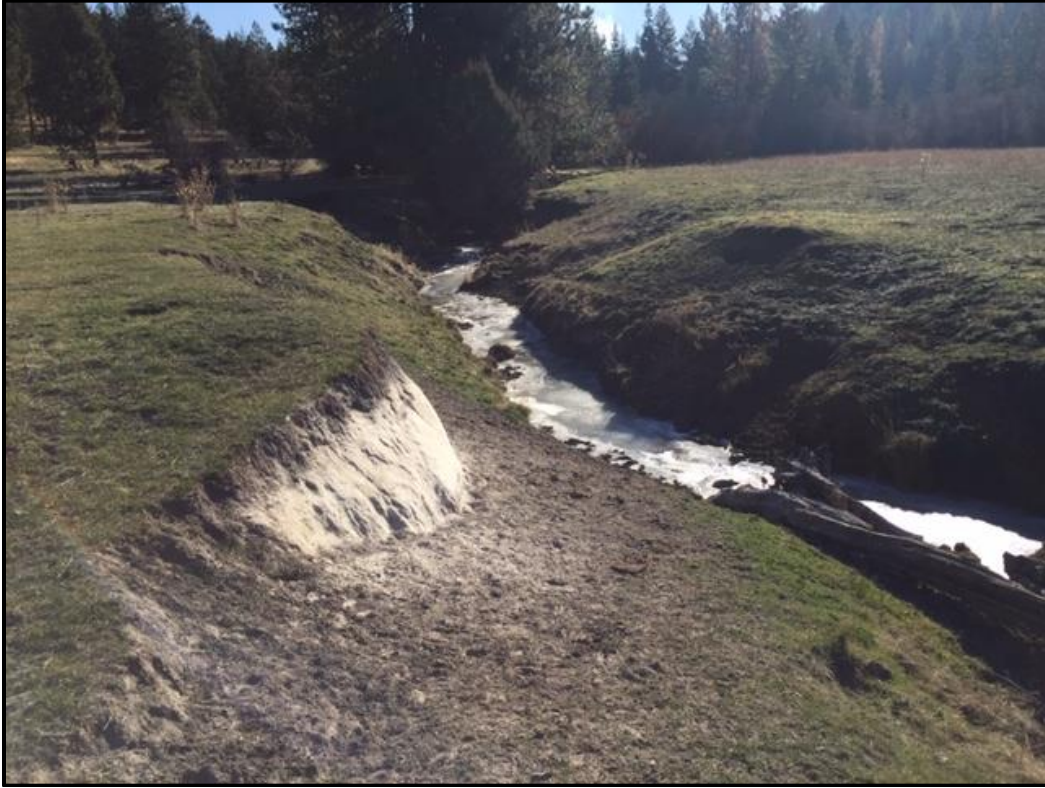
Looking east upstream of Caplinger Creek showing bare soil
