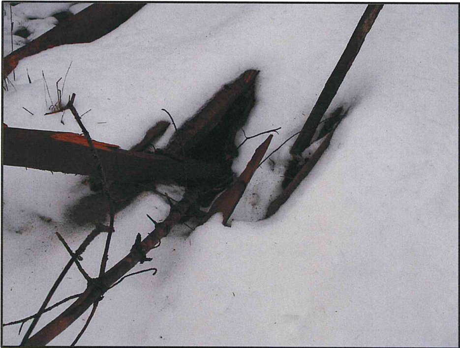
Hole through the deck
