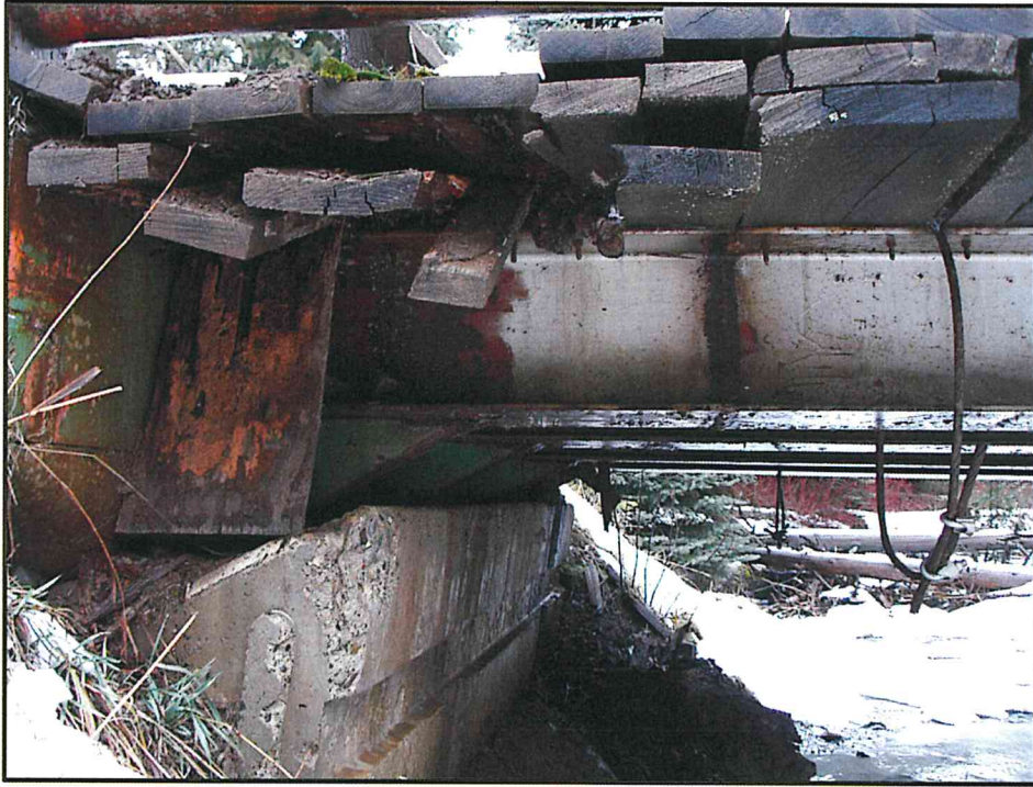
View of damaged decking boards.
