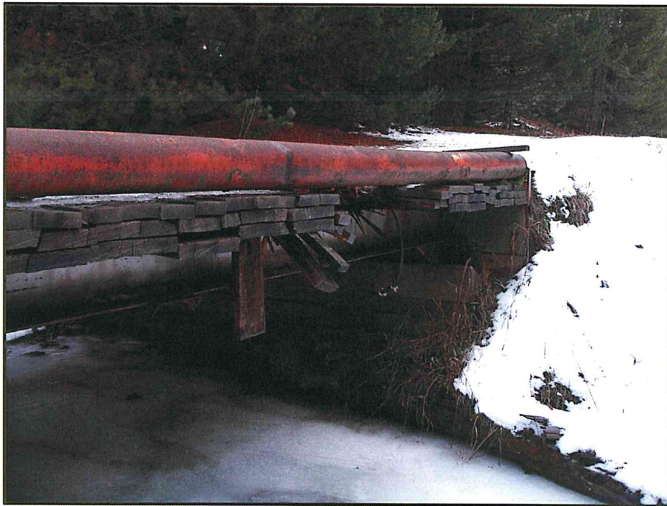
Another view of dilapidated bridge deck.
